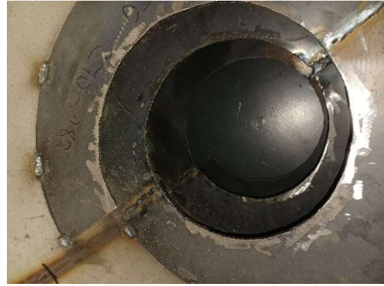
Fig. 8.21 Detail of the helix for spiral flow of flue gases from the constructed pyrolysis reactor
