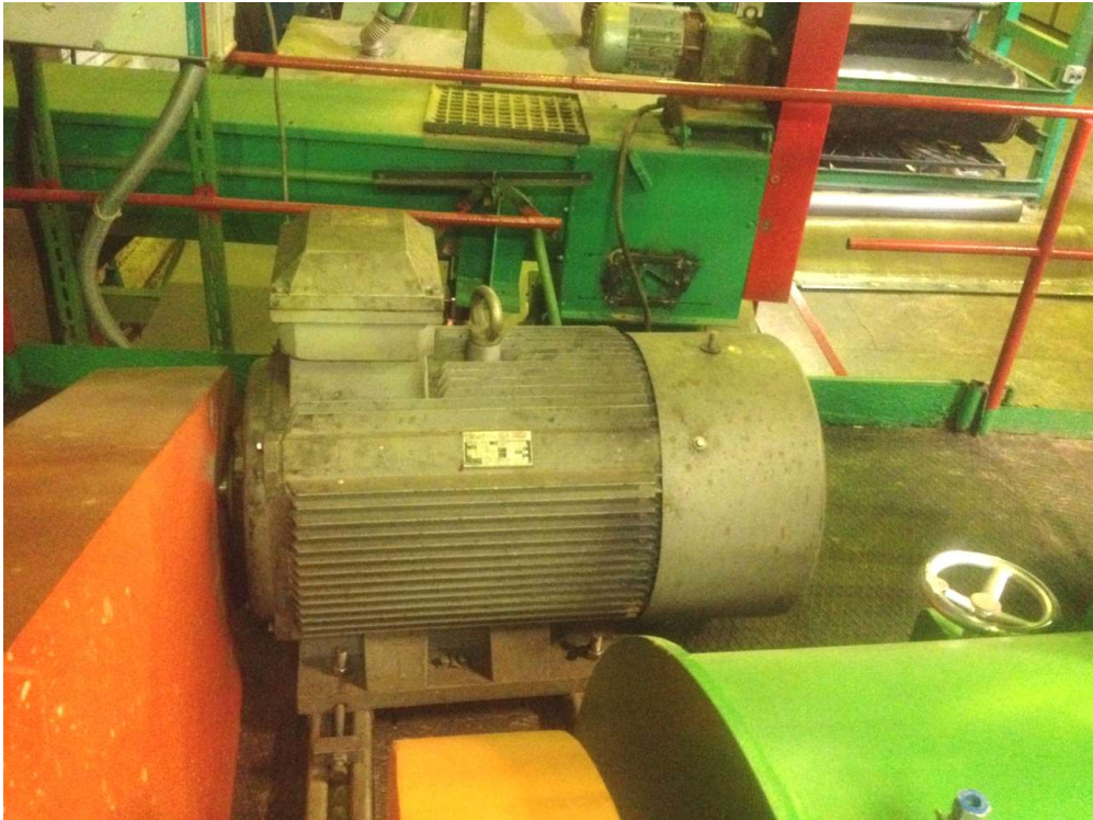
Fig. 4.53 - Thick chip mixer electric motor
