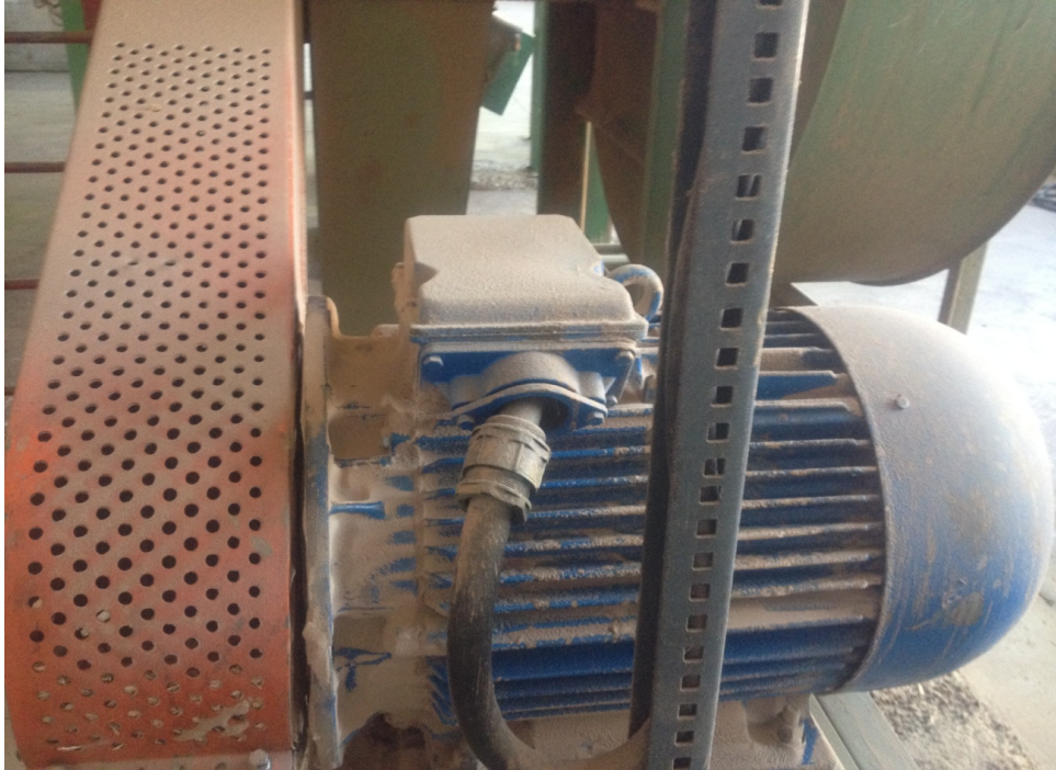
Fig. A.4 - Electric motor of pneumatic classifier
