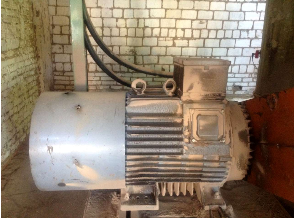
Fig. A.5 - Electric motor of crushing machine
