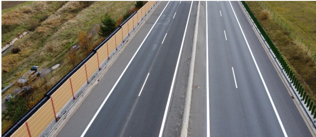
Fig. 3.17 View of the installed noise absorbers in the given section
