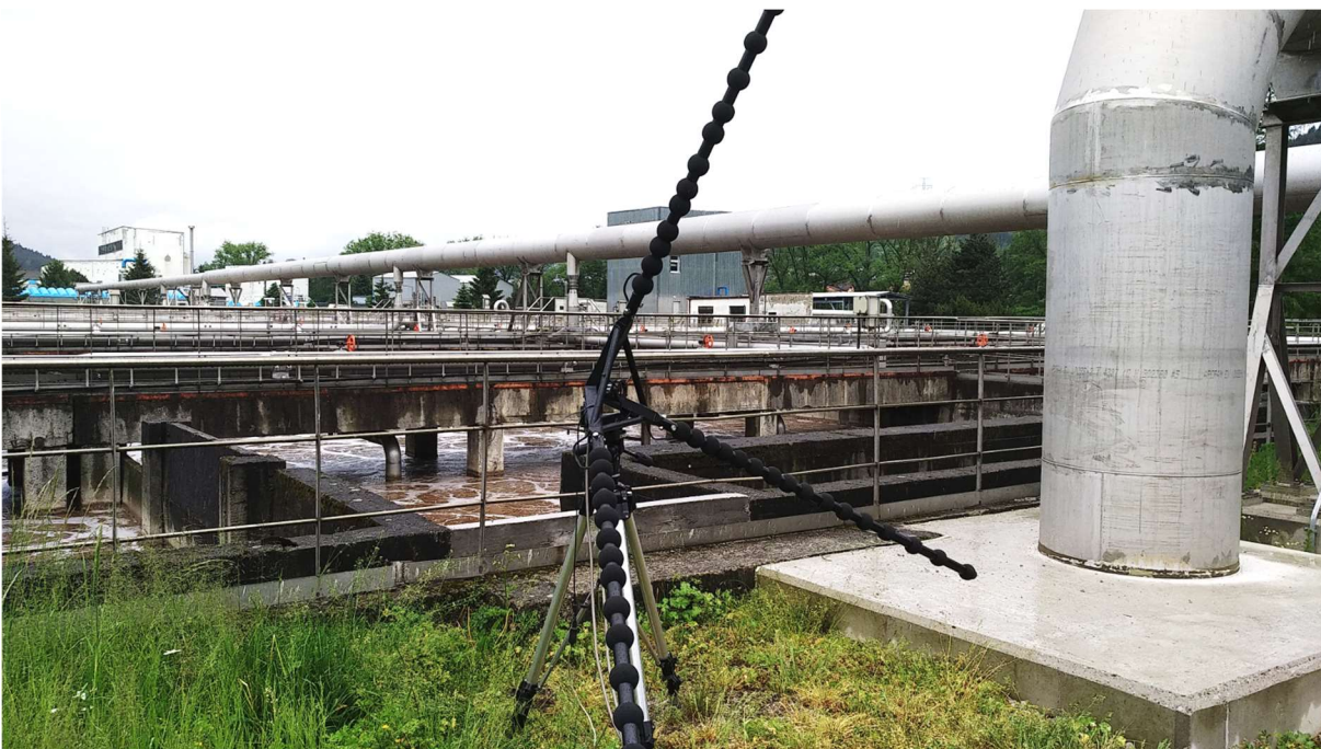
Fig. 239 View of the installed acoustic camera - measurement No. 2
