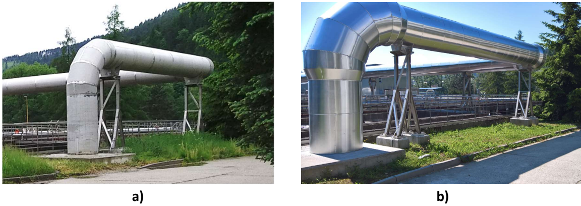
Fig. 249 View of the air distribution pipes (a) before and (b) after application measures.
