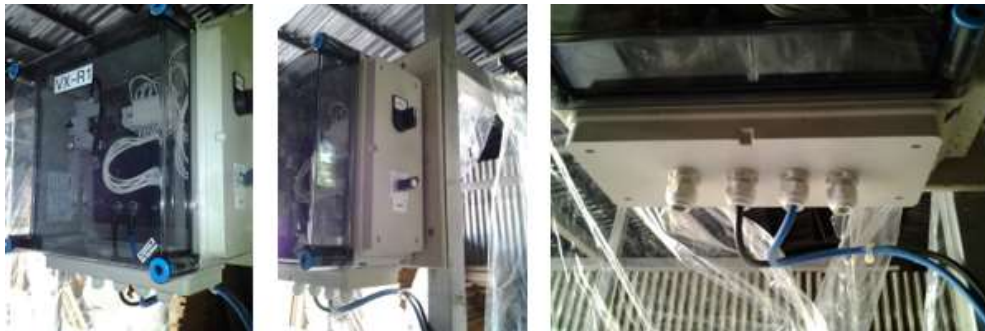
Fig. 223 Real views of the electric motor control box (VX-R1) [123]
